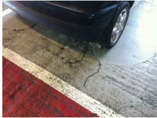
Fig. 2: Cracking and delamination
